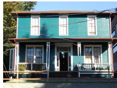
Steele House Apartments were built in 1869 and needed a lead-safe certified contractor to repaint the exterior, funded by CDBG.
