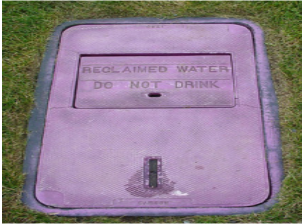
Reclaimed Valve Box
